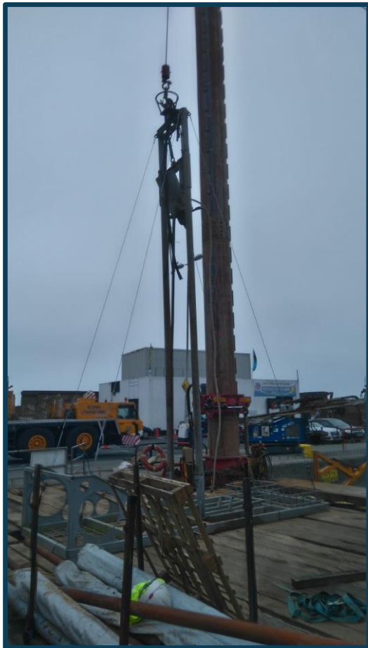
Vibrocore unit set-up on deck of the barge before mobilising to offshore work site
