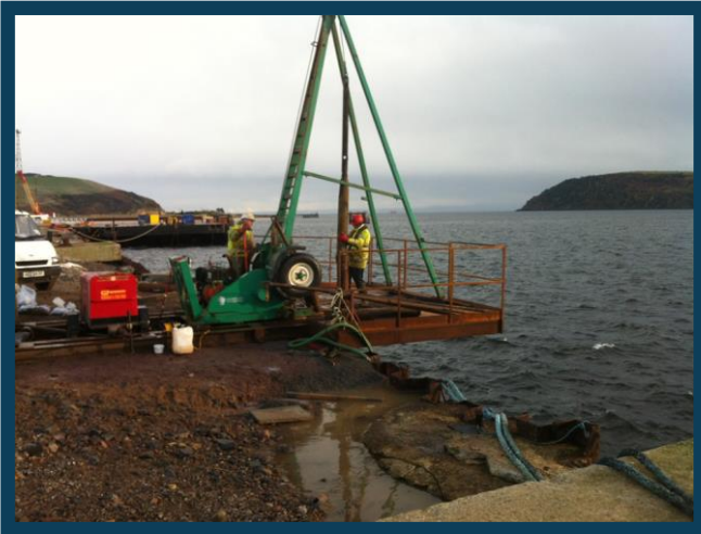
Cable percussion boring rig (Dando 3000) set-up on cantilevered platform for putting down borehole overwater, adjacent to quay wall.
