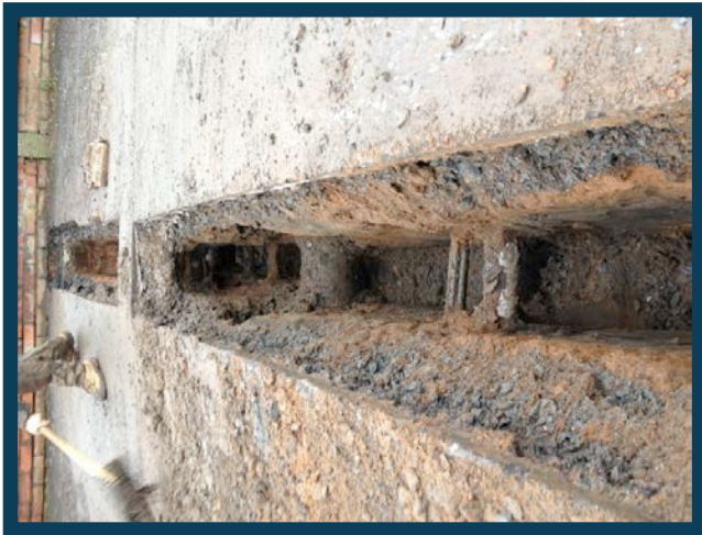
Open section of slit trench, excavated to confirm presence and location of utilities along the scheme route
