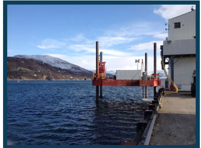
Putting down a borehole adjacent to ice plant on the existing pier
